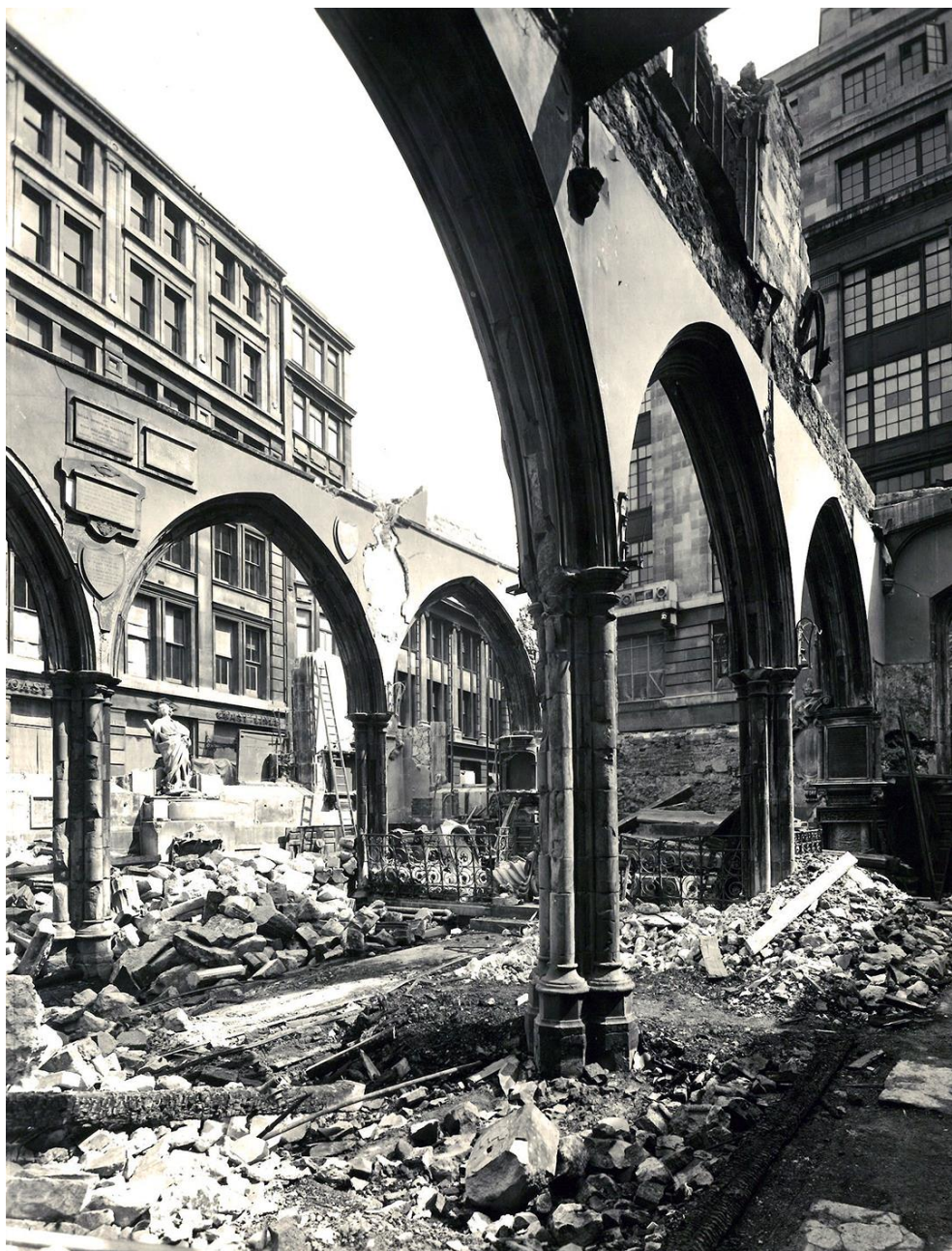
View of the nave of St Olave Hart Street following bomb damage in April 1941
